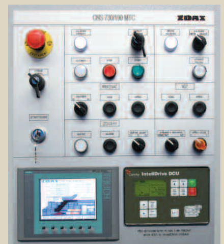
Control system panel with screen
